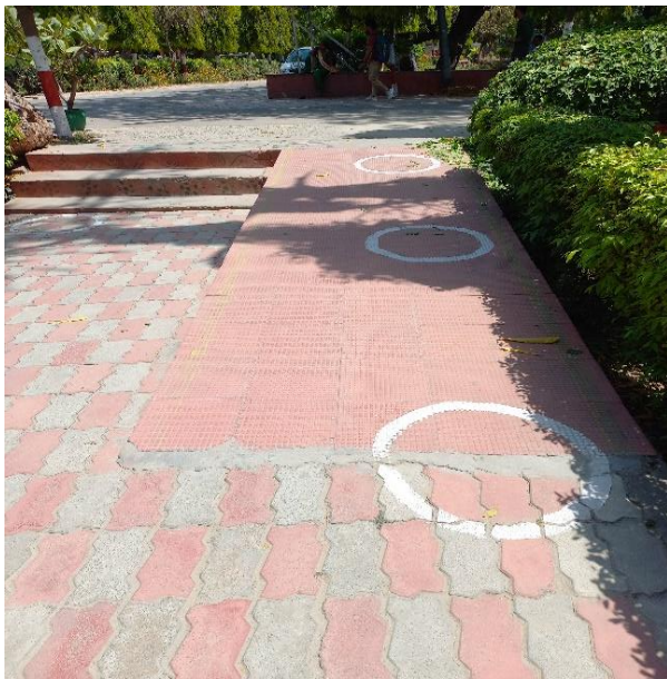
Figure 1.7: Ramp without handrails
